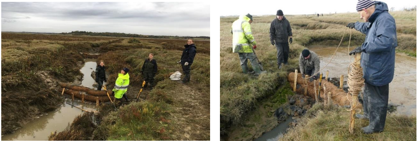
Figure 5 Environment Agency and Essex Wildlife Trust installing the Moverons structures (left); Essex Wildlife Trust volunteers installing structure at Abbots Hall nature reserve (right). Both in November 2018.
