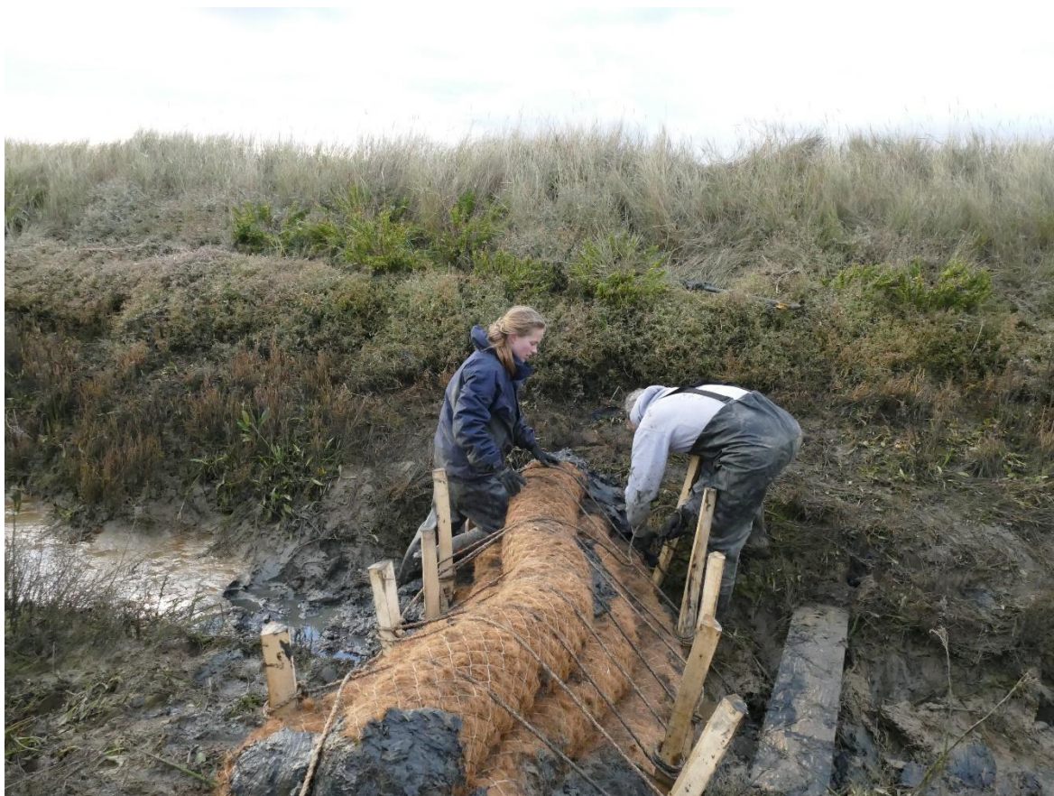
Figure 3 Coir rolls being installed as a 6-roll structure at Abbotts Hall by an EWT staff member and volunteer, November 2018
